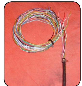
End of Cable Opening
